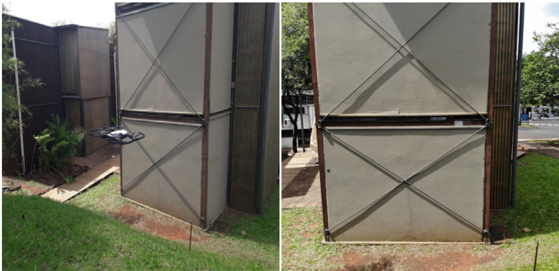
Figure 6: Drone Mavic Air 2 capturing the façades of Unit 001 (Left), Photo captured (Right). Source: Elaborated by the Authors (2022)
