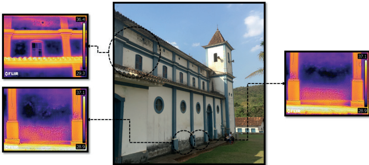
Figure 11 – Areas of moisture concentration on the left side of the church. Source: Authors' collection.
